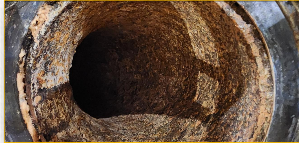
Picture showing pipe internal corrosion in a Potash Mill
