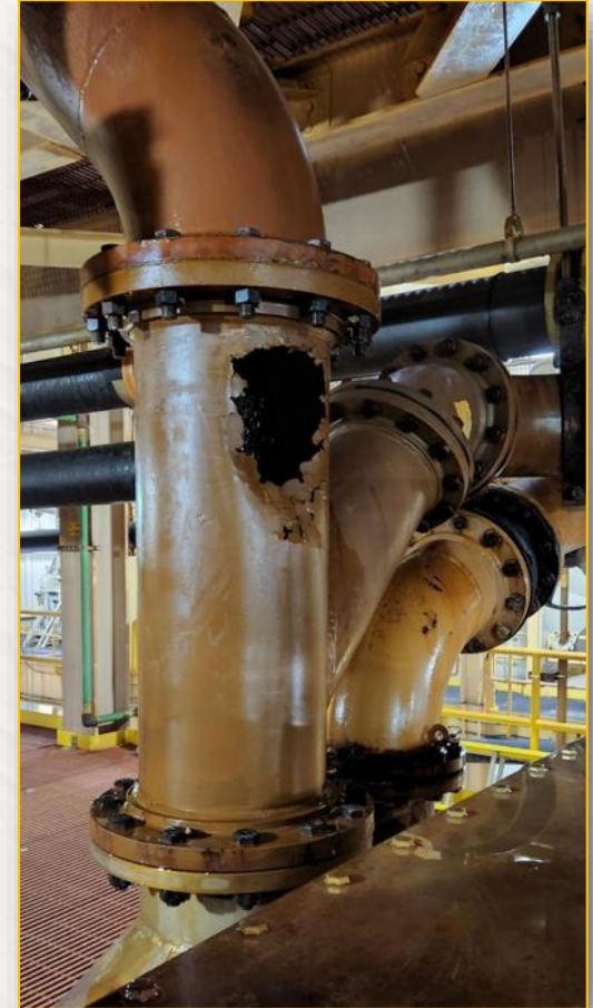
Picture showing pipe wear in a Potash Mill
